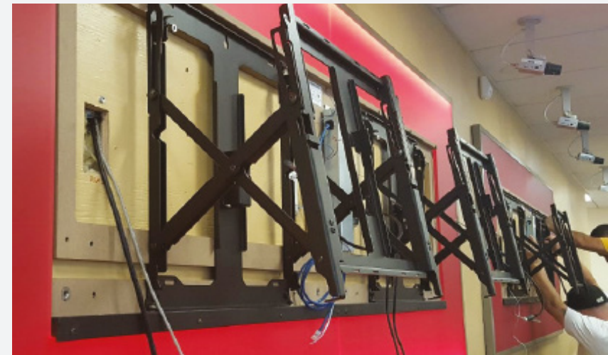
Our electrical services provide robust code-compliant wiring and installation, all while powering CCTV surveillance systems tailored for your facilities' security solutions.
