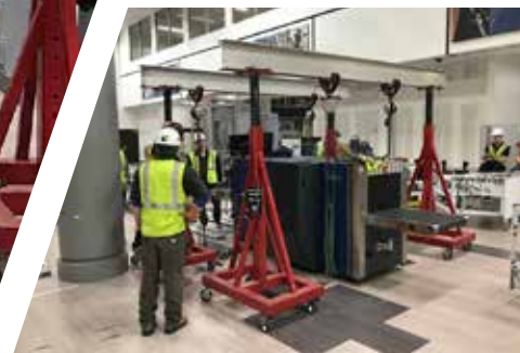
AUTOMATED SCREENING LANES (ASL) OEM > MacDonal Humfrey, Vanderlande, Scarabee
